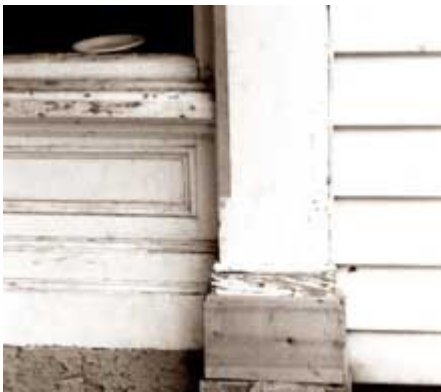
Rather than replace an entire wooden storefront, a new wooden component can be pieced-in, as seen in this column base. Photo: NPS files.
